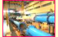
Calibration of Bypass flow meter
