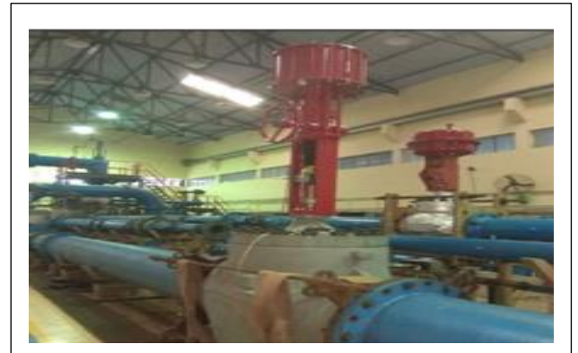
Testing of 600 mm Valve at WFL
