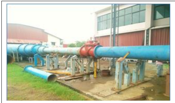
Cv testing of a Swing check valve at LWFL
