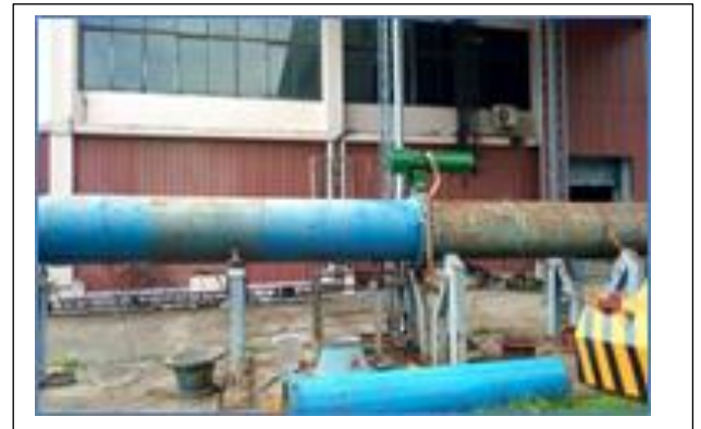
CV testing of a Butterfly Valve at LWFL
