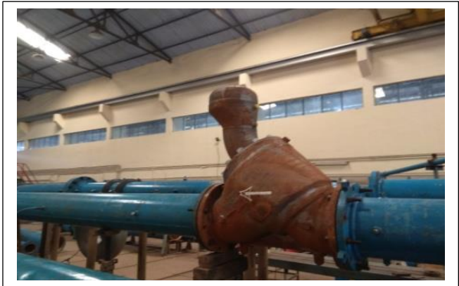
Surge Relief Valve under test
