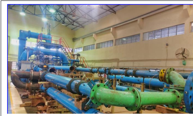
Change-Over Valve under test
