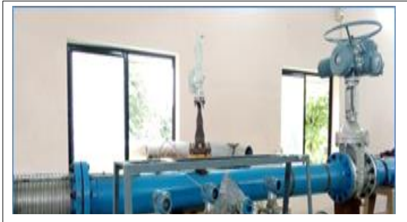
Safety Relief Valves under testing at FL Test Facility
