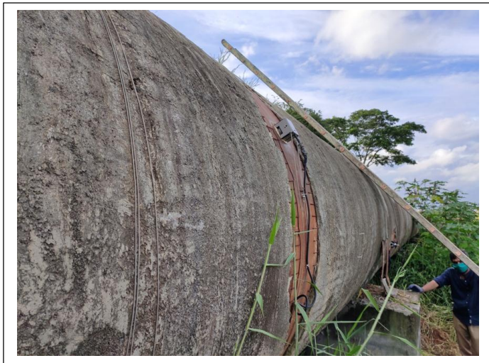
2400mm Ultrasonic flow meter Calibration.
