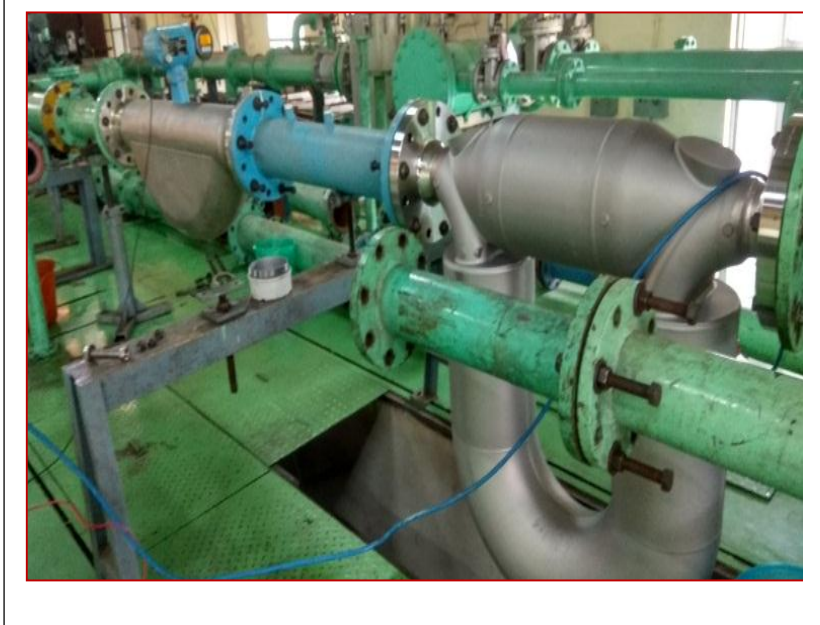
Mass flow meter of size 8" calibration at Oil Flow Laboratory.
