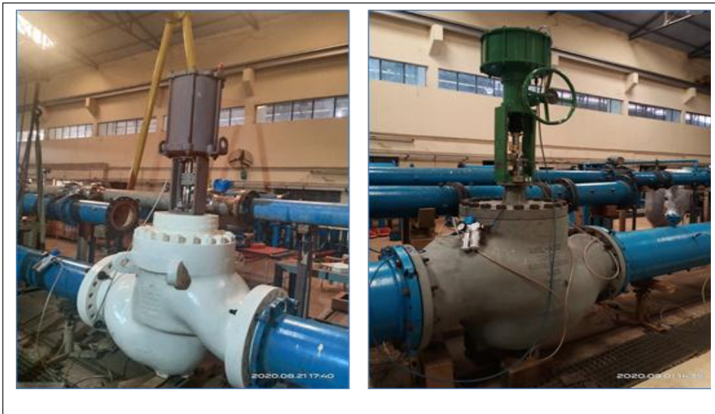
Testing of control valves at WFL
