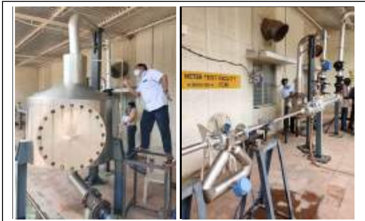
On-site calibration of reference volume tanks and certification of water meter test facility of NTADCL at Tirupur, Tamilnadu.
