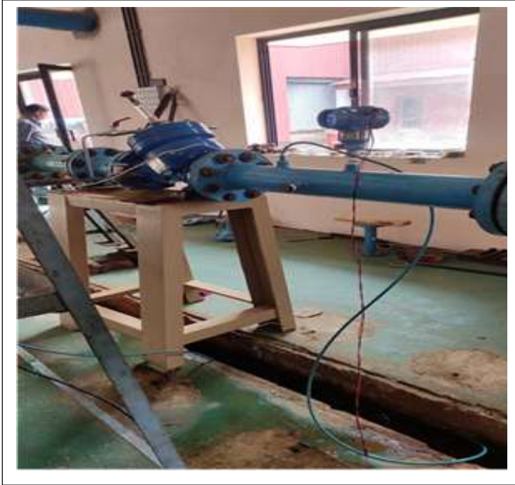
Performance test of 4" Valve at VCRC
