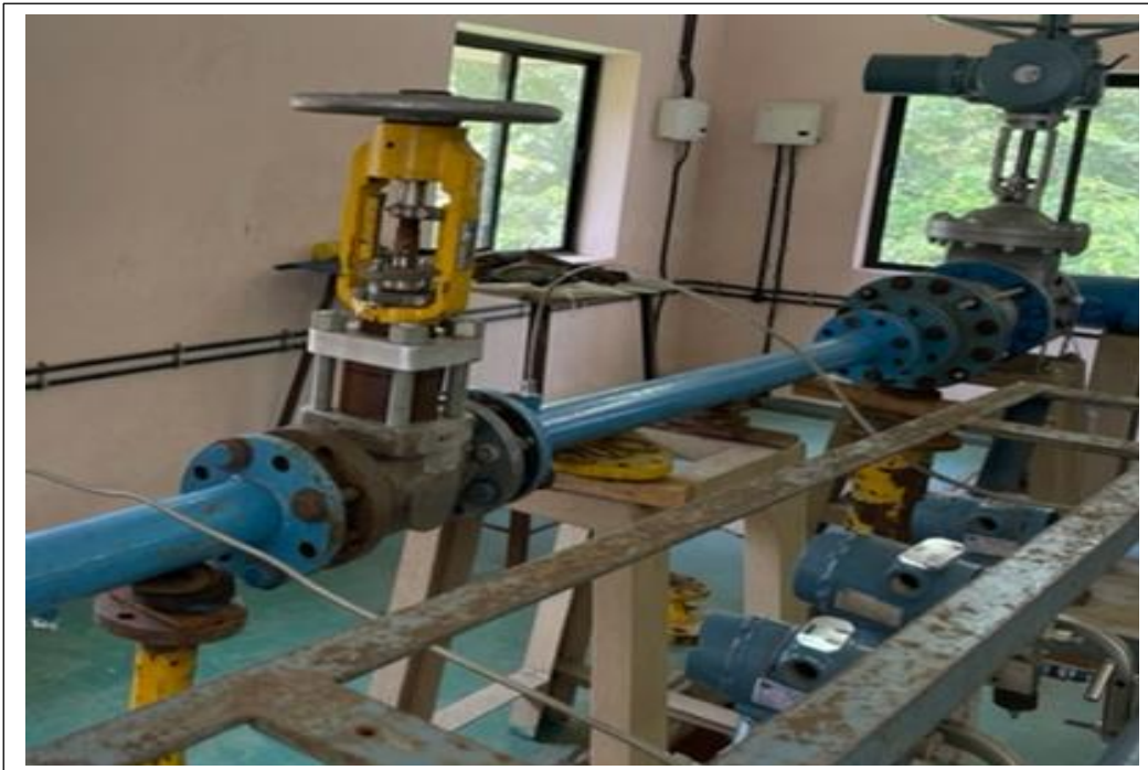
FL testing of valves of sizes 4” at LWFL
