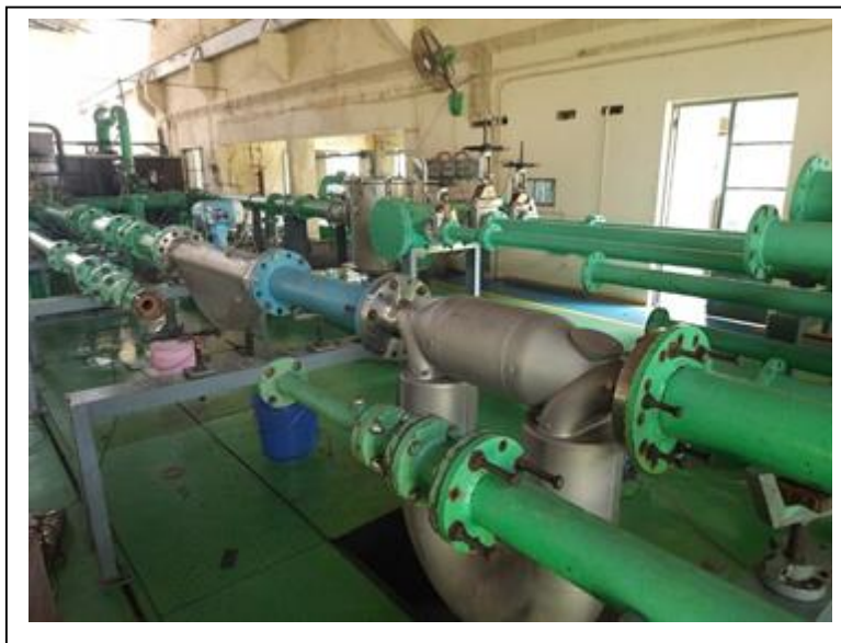
Mass Flow Meter Calibration at OFL
