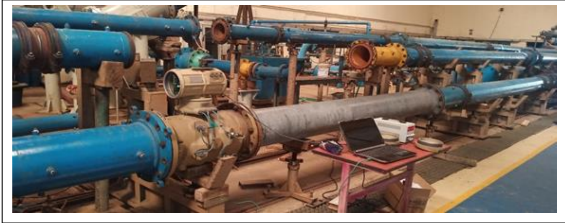
Calibration of inline ultrasonic flow meters of size 12”at WFL
