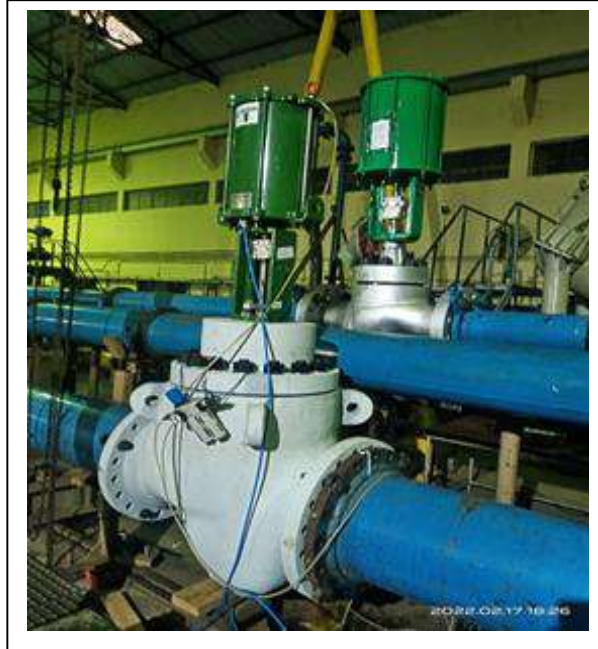
Testing of 20" valve at WFL
