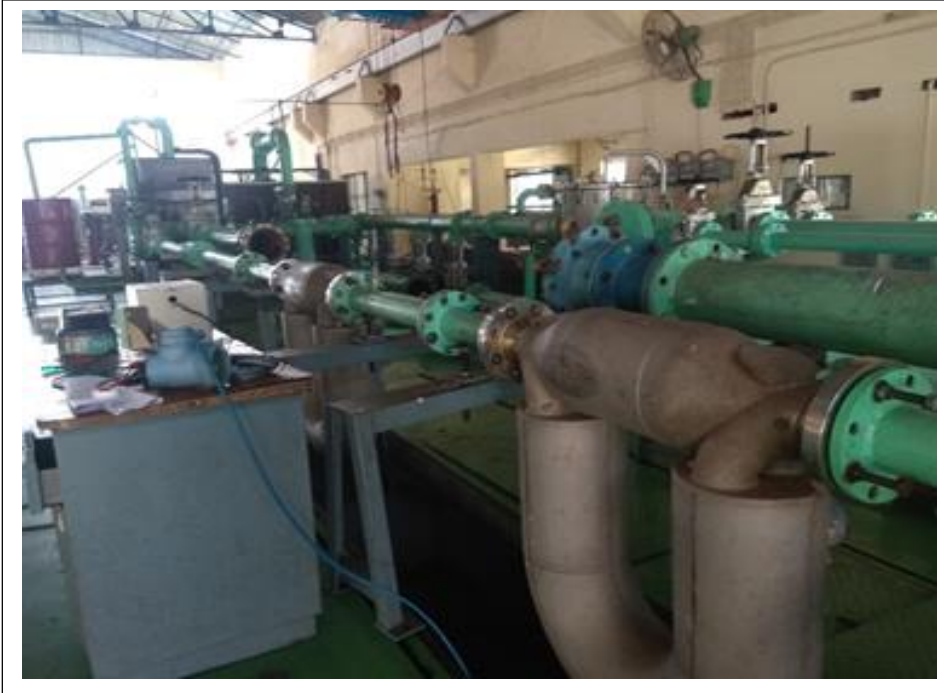
Mass flow meter of size 6'' calibration at Oil Flow Laboratory
