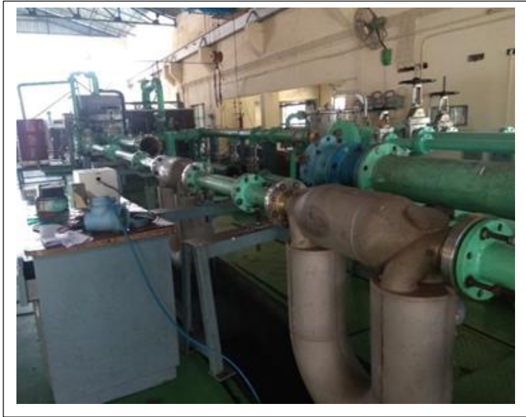
Calibration of mass flow meter (Size 6") at OFL
