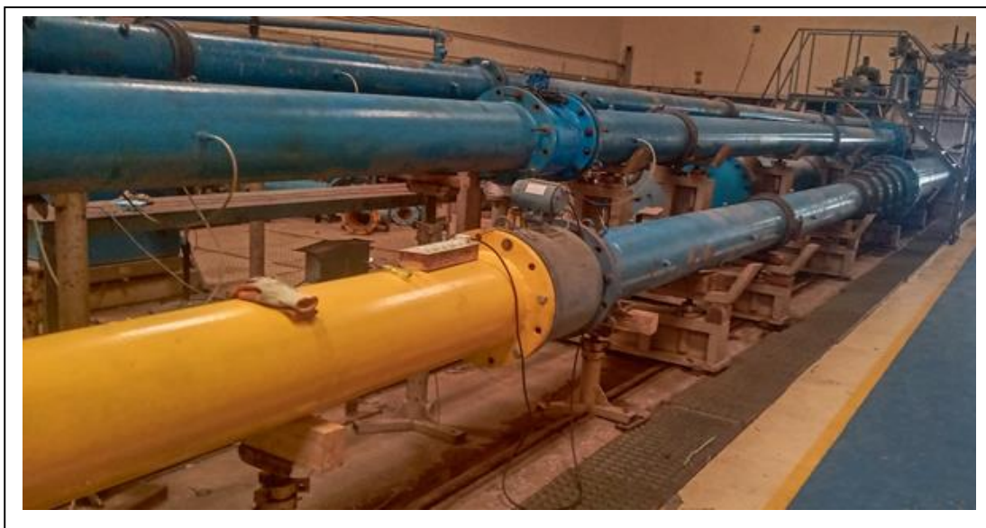
Calibration of 16" magnetic flowmeter at WFL
