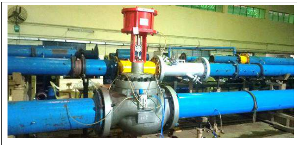
Testing of 18" valve at Water Flow Laboratory
