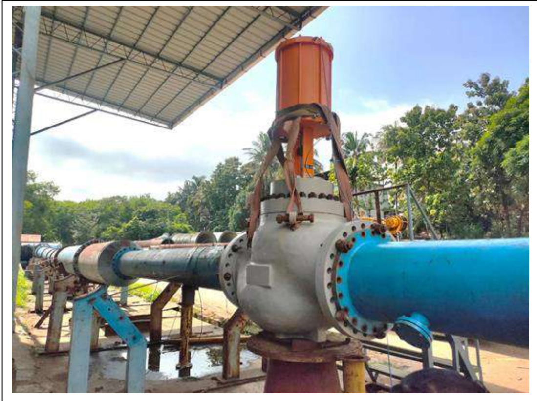
Testing of 600 mm Control Valve at LWFL
