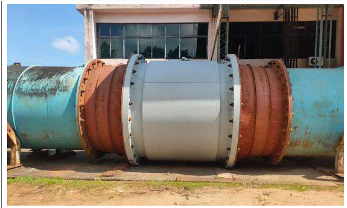
Calibration of 3000 mm Electromagnetic Flowmeter at LWFL
