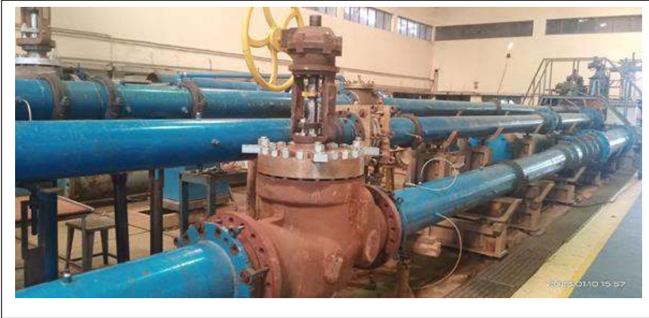
Testing of valve of size 16" at WFL
