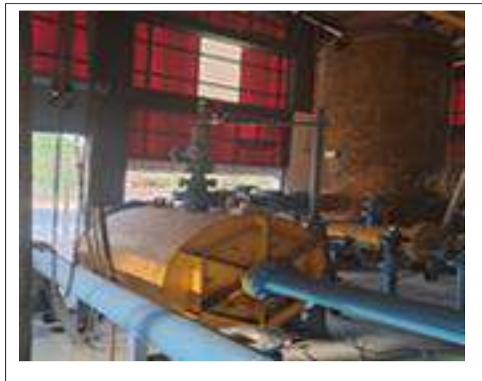
Testing of Safety Valve at HPATF
