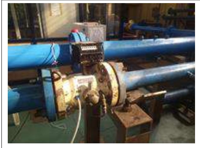
Calibration of Turbine Flow Meter at HPATF
